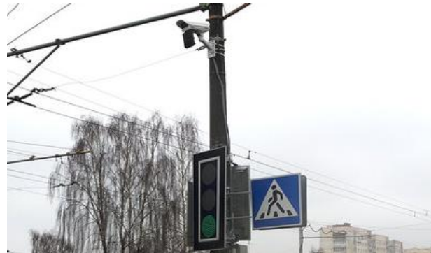
Figure 6. Placement of the video module on the street lighting support.
