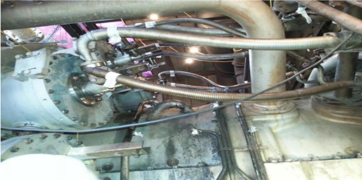
Figure 13 Assembly of pipes connected to the combustion chambers
