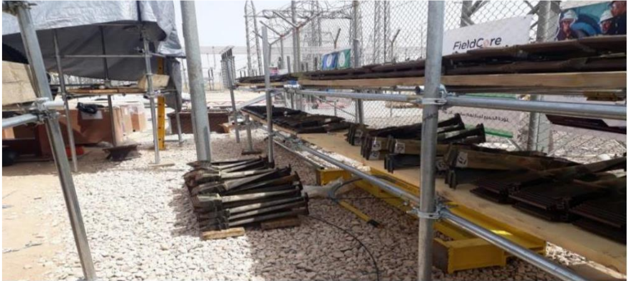
Figure 5 Old turbine blades for the three stages
