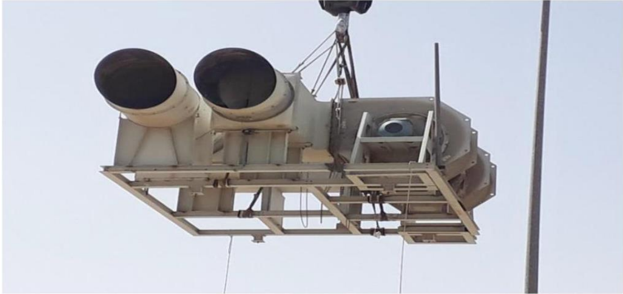
Figure 1 BT fans with air ducts
