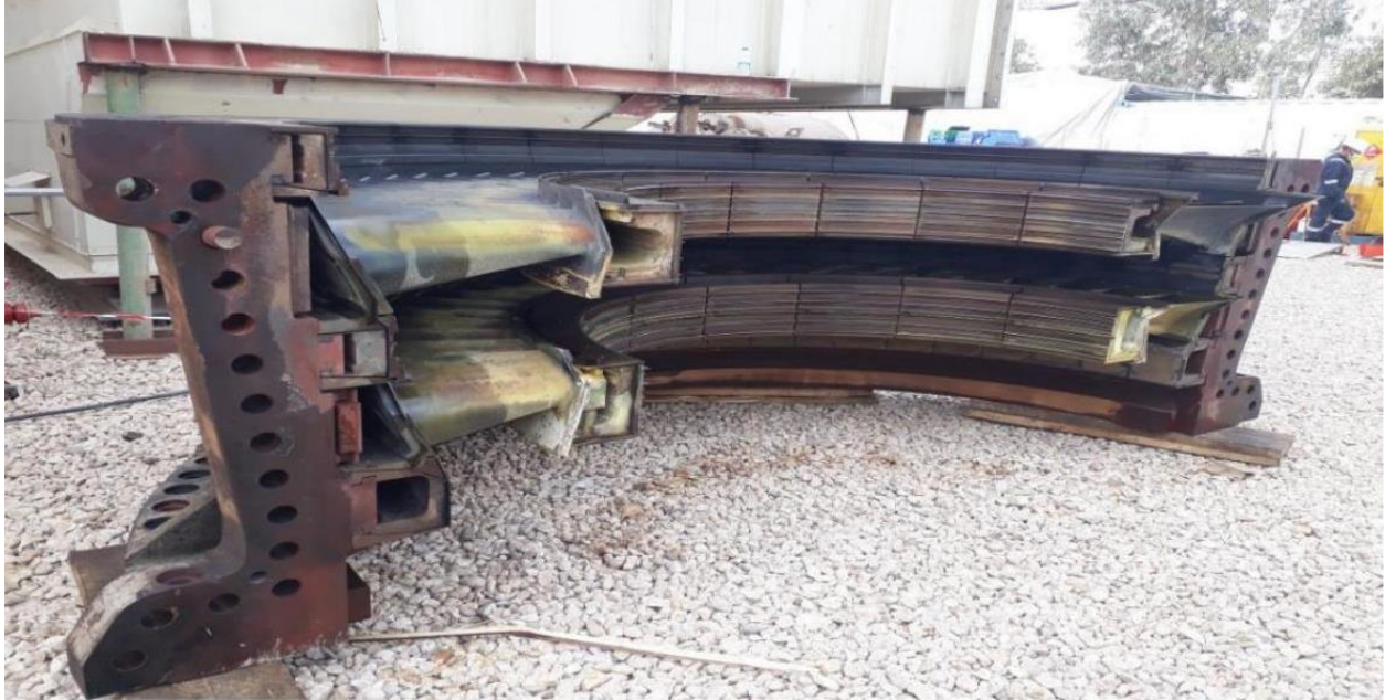
Figure 4 upper turbine cover with old internal parts
